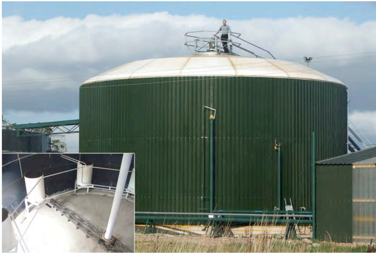
Digester showing input tank (l), CHP enclosure (r) and mixing system (inset)
