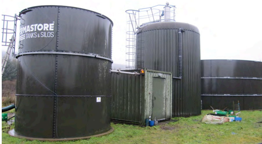
Installation showing input mixing tank on left, control kiosk, digester tank and post store
