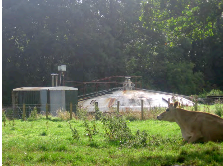
Digester showing boiler/control/separator kiosk on left and digester tank on right.
