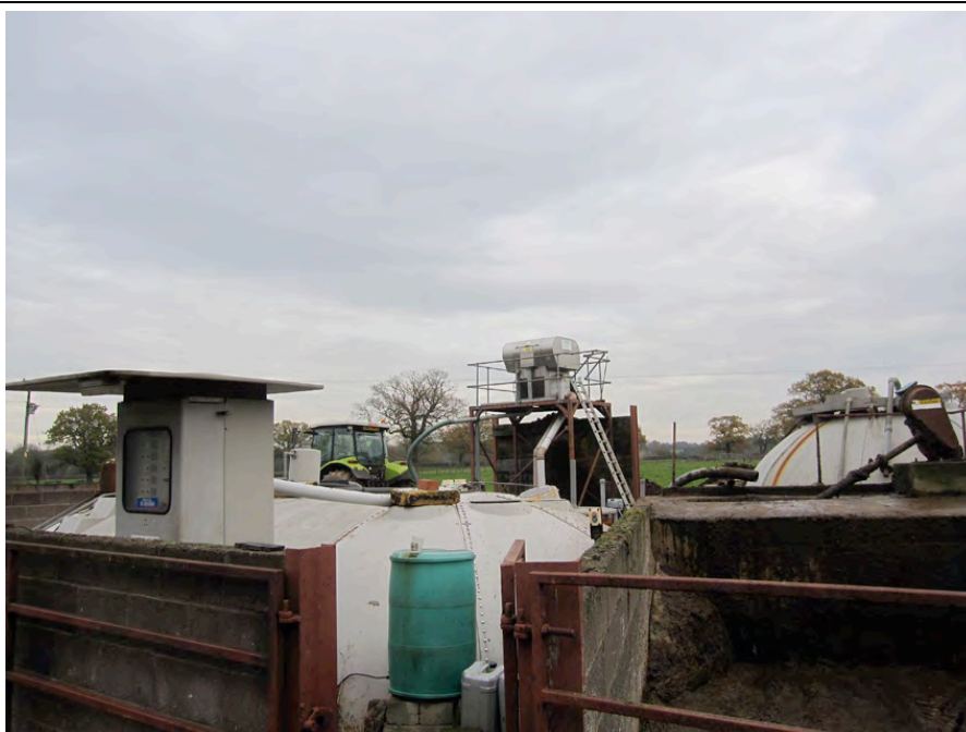
Hill Farm digester with control kiosk in foreground, loading pit on right, with loading auger behind, digester behind kiosk, elevated separator in the background and second digester on the right hand side in the background.
