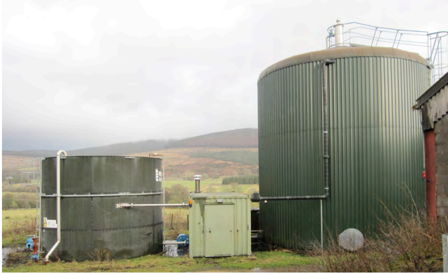
From l to r: Input tank, control kiosk and (out of picture) digestate storage tank
