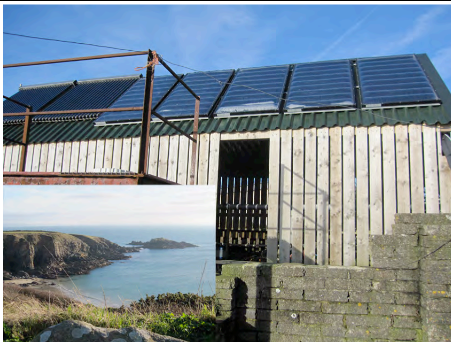
Digester shed showing thermal solar installation on top and (inset) beautiful Caerfai Bay
